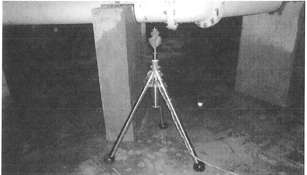
Figure 2. The PAX Water Mixer was installed in a 5MG tank with an existing passive mixer (shown behind PAX Water Mixer in above image).
